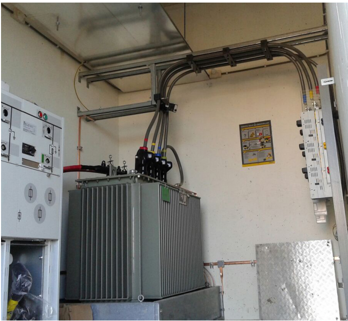
Middle voltage transformer with multi-layer redirection construction
