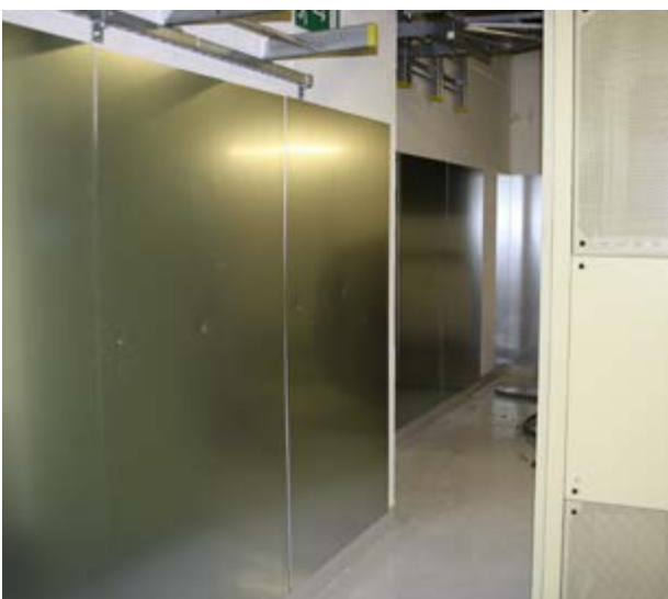
MuFerro afscherming distributiestation
