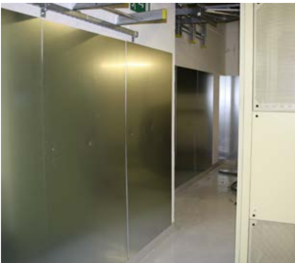
MuFerro shielding of a power distribution station
