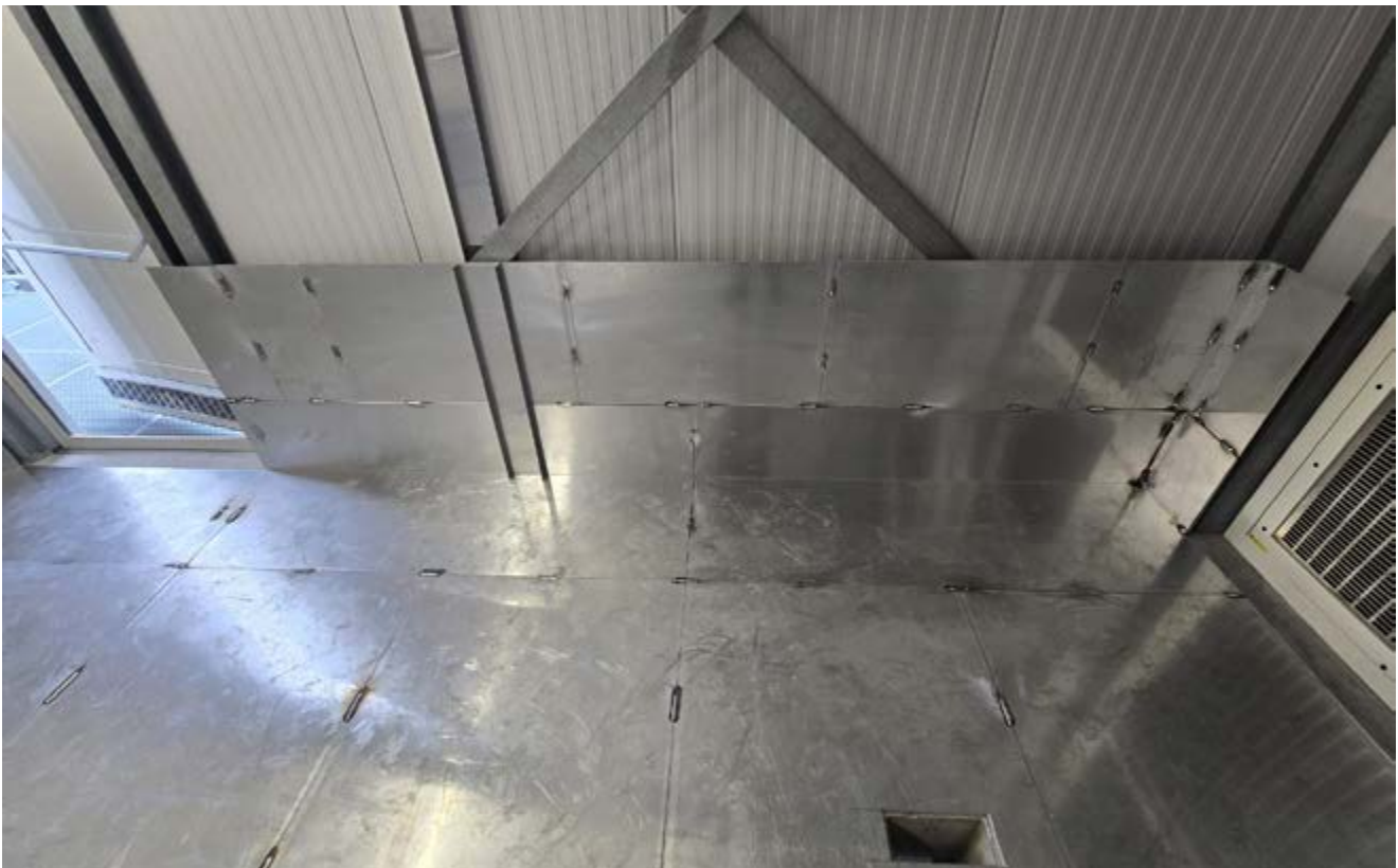
Shielded floor in a transformer room on the roof.
