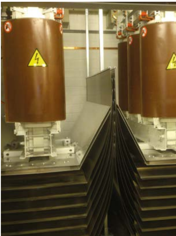
Indoor transformer room with electromagnetic shielding
